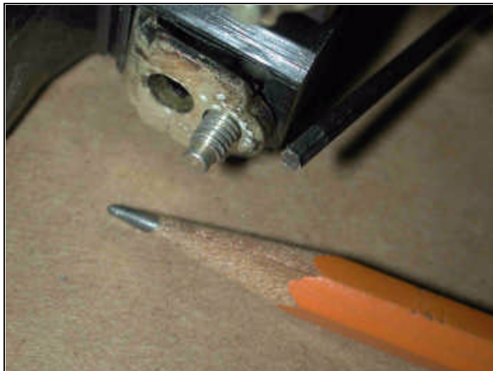
FIGURE 7 - ONE LOAD-SIDE CONTACT AND ITS 8-32 CLAMPING SCREW, ON THE FPE 100-AMP MAIN BREAKER OF FIG. 6. THE SCREW-HEAD TAKES A 3/32" ALLEN WRENCH, WHICH IS ONLY SLIGHTLY LARGER THAN THE LEAD OF THE #2 PENCIL. (The larger hole provides clearance for the screw protruding from the stab contact plate)
