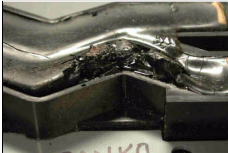
FIGURE 3 - OVERHEATING AT THE CONTACT BETWEEN THE BUSSBAR AND THE STAB SOCKET ASSEMBLY CAUSED THIS DAMAGE TO THE INSULATION.
