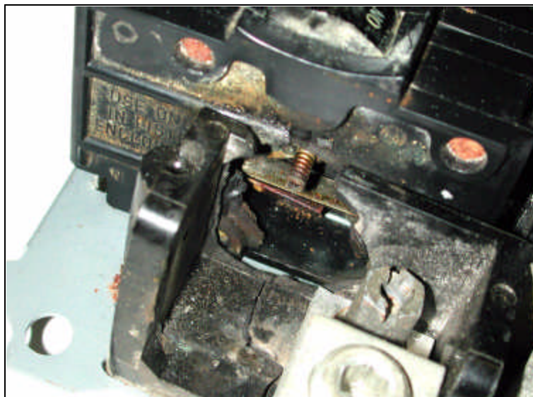
FIGURE 9 - VIEW DOWN TOWARD UPPER RIGHT OF PANEL SHOWN IN FIG. 8. THE FPE STAB-LOK® TWO-POLE 30-AMP BREAKER FED THE CLOTHES DRYER.
